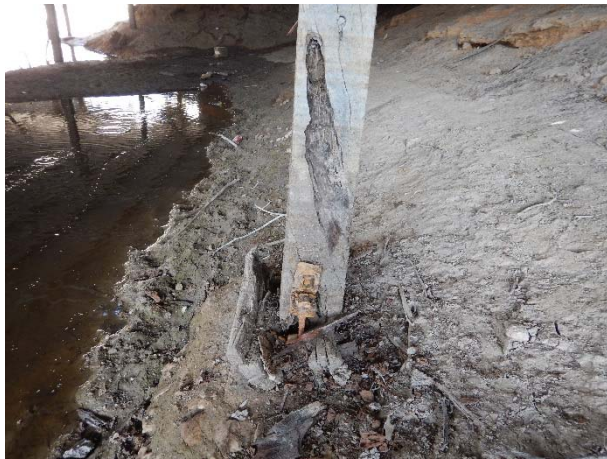
Photograph M: Rotten timber column and corroded connection bolt.
