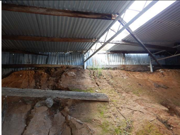
Photograph EE: Formation of rills and gullies in embankment. Broken purlins and missing sheeting.
