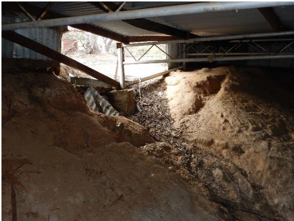
Photograph G: Eroded embankment, undermined steel post and concrete footing
