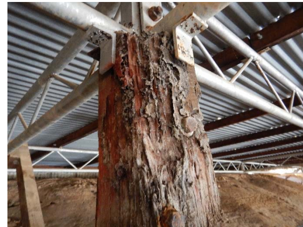
Photograph N: Termite damage on upper portion of timber column. Significant loss of 20% section thickness.
