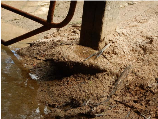
Photograph I: Eroded base soil of concrete footing.
