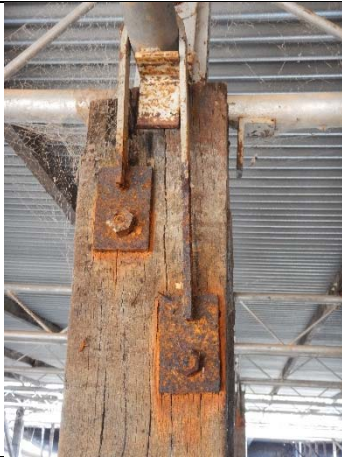
Photograph Y: Light corrosion on strap and bolts connecting the roof truss and timber column
