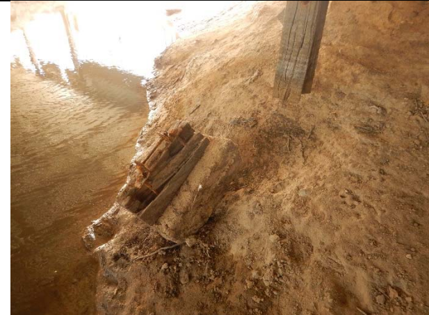
Photograph FF: Completely washed out concrete footing.
