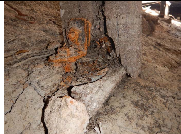
Photograph R: Fully rotten and split base timber, badly corroded anchor and connection bolt
