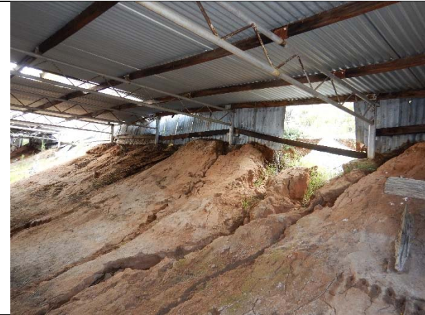
Photograph DD: Formation of rills and gullies in embankment
