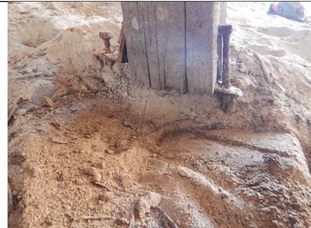
Photograph T: Total deterioration of base timber and corroded bolts and anchors.
