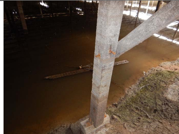
Photograph V: Timber bracing appeared to be missing from the column.
