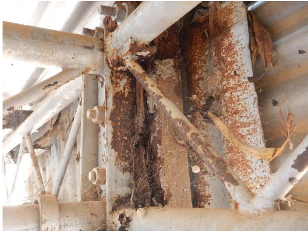
Photograph K: Corrosion of truss and sheeting, termite damage on timber packer
