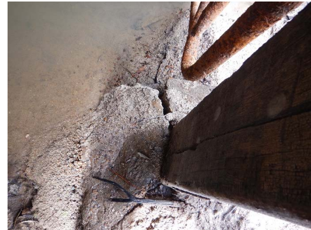
Photograph H: Wide crack to concrete footing
