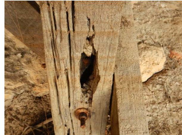
Photograph L: Rotten timber column, termite damage and corroded connection bolt.
