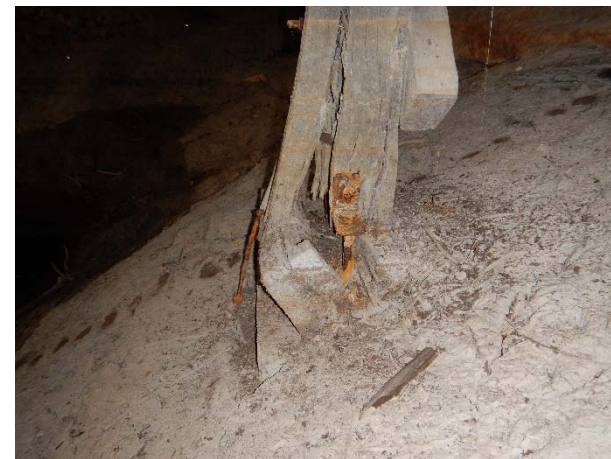
Photograph P: Typical wide splits and delamination of lower part of column. Rotating base timber
