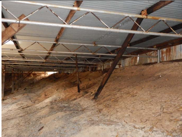
Photograph U: Fallen timber purlins.
