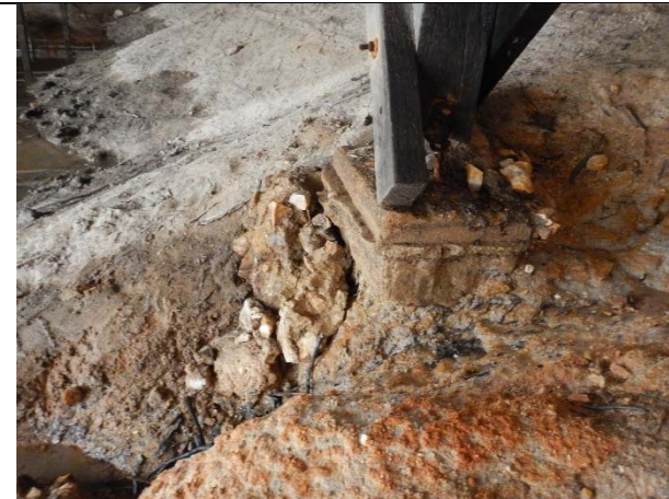
Photograph BB: Erosion of soil below footing
