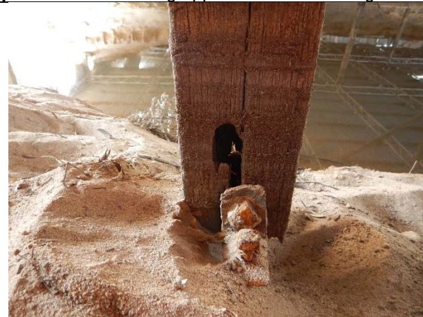
Photograph X: Badly corroded anchors and connection bolts, hole in timber column
