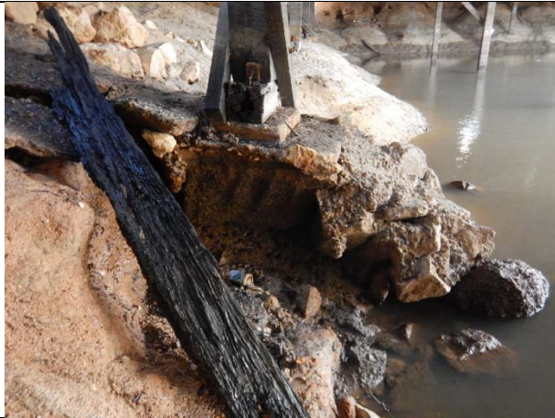
Photograph CC: Eroded soil around footings
