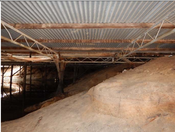
Photograph AA: Corroded gutters.
