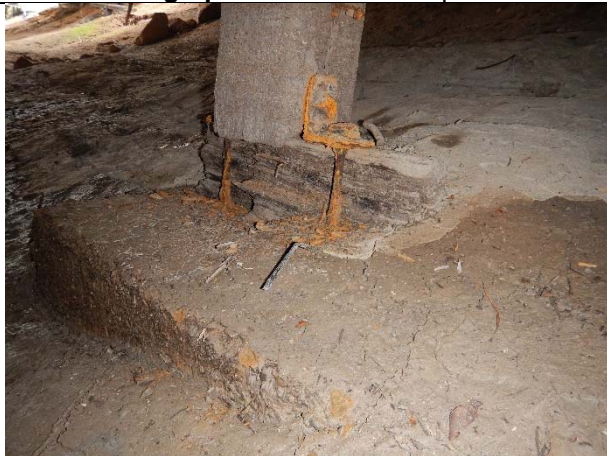
Photograph W: Badly corroded anchors and connection bolts
