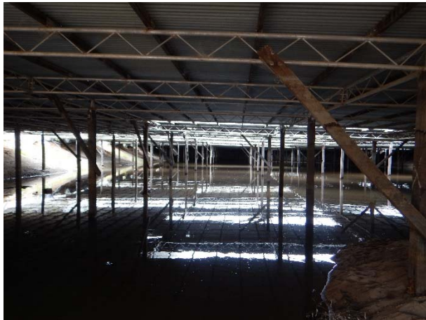
Photograph C: Internal support columns submerged in water.
