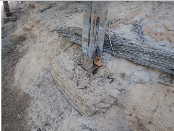
Photograph S: Total deterioration of base timber and corroded bolts and anchors.
