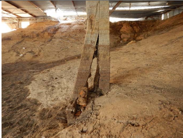
Photograph Q: Typical wide splits and delamination of lower part of column. Moved base timber
